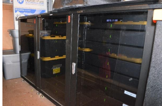
Fig.3. HI-SEAS battery bank. Photo credit: Ansley Barnard.
