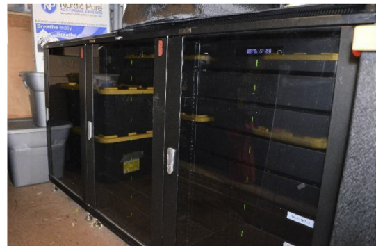
Fig. 3. HI-SEAS battery bank. Photo credit: Ansley Barnard.
