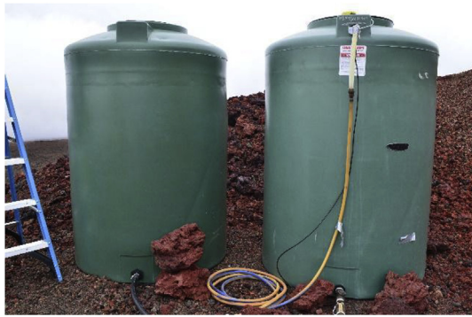
Fig. 5. HI-SEAS external water tanks containing 3785 L (1000 gallon) of water. Photo credit: Ansley Barnard.
