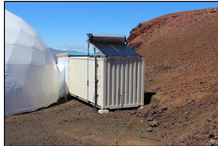
Figure 9: The 150 gallon solar water heater. Photo Credit: Simon Engler
