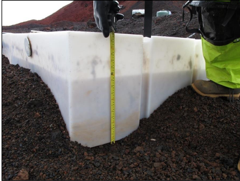
Figure 5 The 500 gallon (1893 L) septic tank being manually measured for its current capacity. Photo Credit: Dr. Sian Proctor
