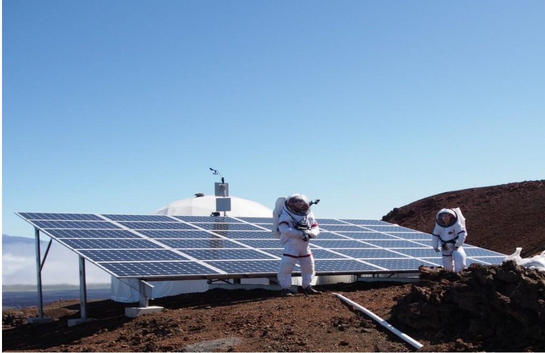
Fig. 2. HI-SEAS 10-kW solar array.
